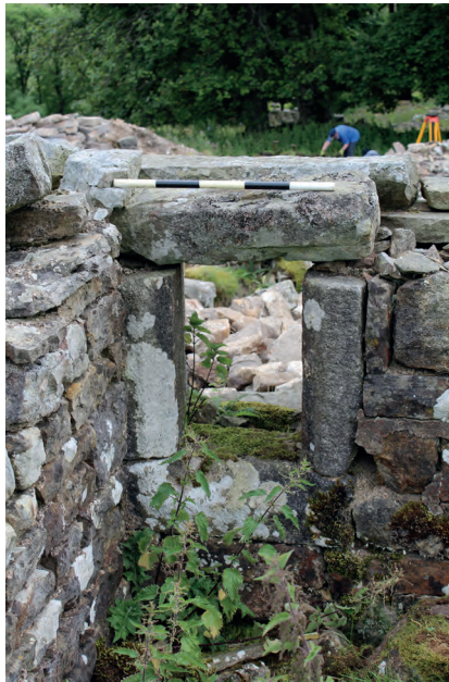
Figure 13 Surviving window in the north wall with chamfered surround. The wall of the later rear outshot abuts the main structure wall, masking part of the window jamb
